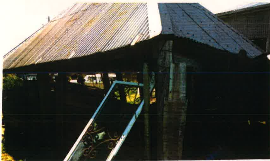
Photograph showing replacement strips of tin used to hold up spouting.
